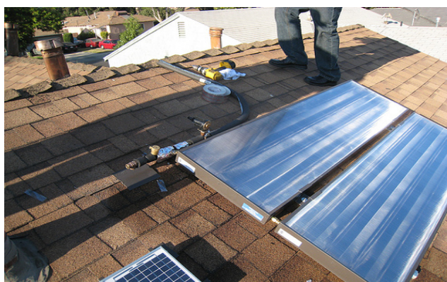
Solar Collectors mounted in position. The PV solar panel for the circulation pump is visible in the foreground.
