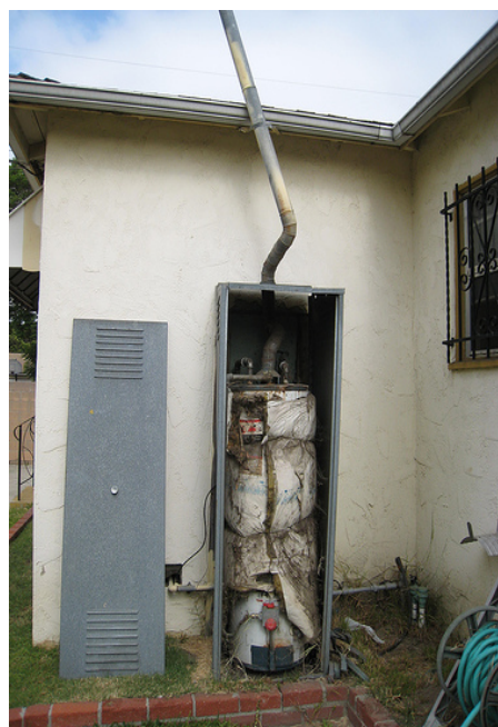
40 gallon tank and enclosure before installation.
